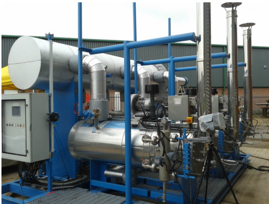
Fig. 4: Pilot unit - three-burner thermosyphon preheater.
