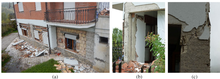
Fig. 2 Damage to RC buildings a, b very heavy damage to masonry infills, c shear failure in column, building ID 12 Lat 42,37,33.198N, Long. 13,17,25.944; source EEFIT (2016)
