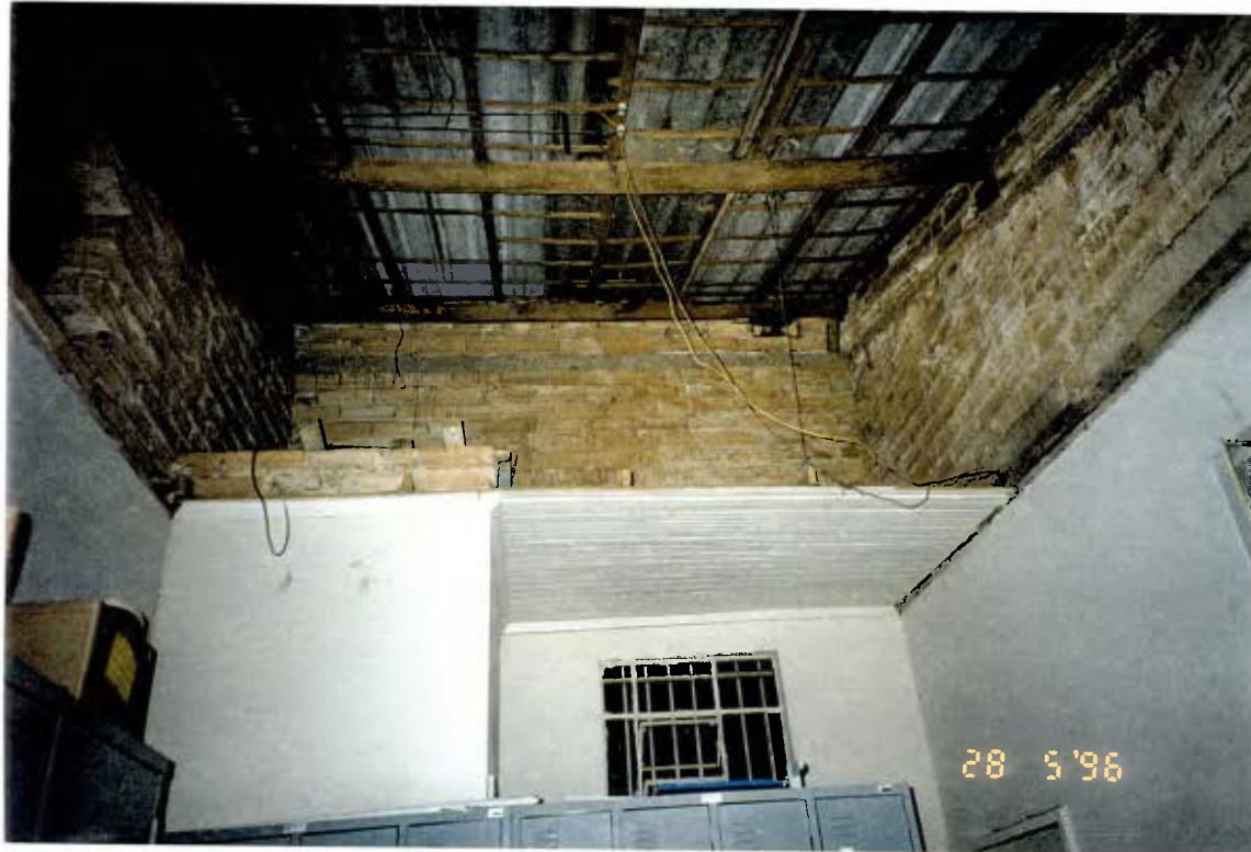
Figure 4.2- Photos showing the staff room and one of the classrooms in school 1. Note the very poor conditions of the ceiling (which fell down the year following the first visit), the conditions of the wall and the size of the windows. There was little circulation of air and, in the summer, the environment was suffocating.
