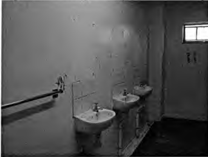
Image 32: 06K03d: Simunye Secondary: Girls' cloakroom with graffiti and mirrors missing
