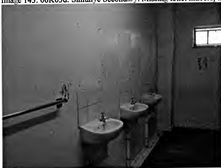
Image 143: 06K03d: Simunye Secondary: Missing toilet mirrors, and wall graffiti
