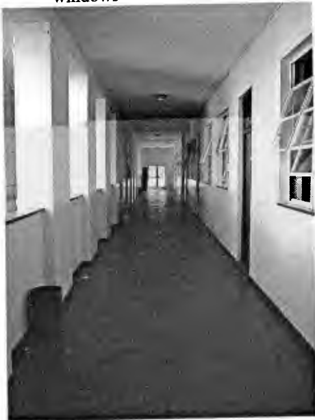
Image 11: 03K17i: Centenary High: 1930s block, corridor open to the elements and with classroom sash windows
