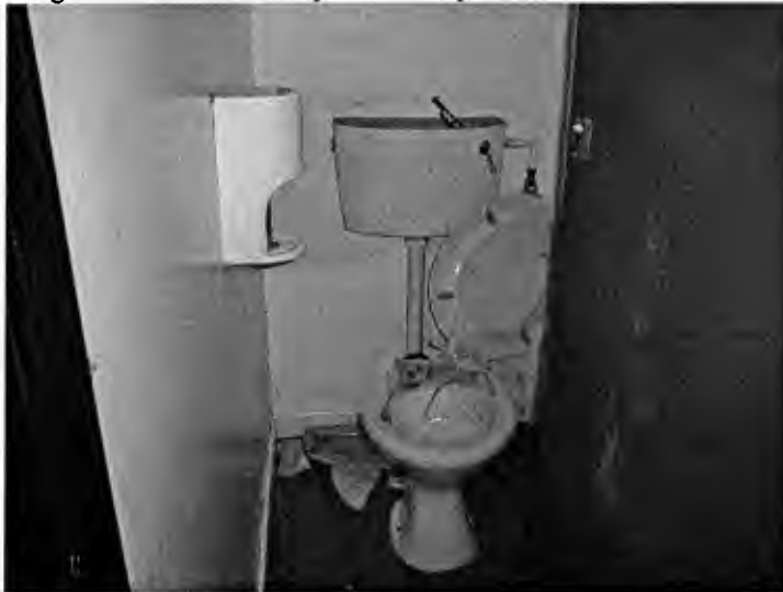
Image 33: 06K03f: Simunye Secondary: Smashed toilet bowl and cistern
