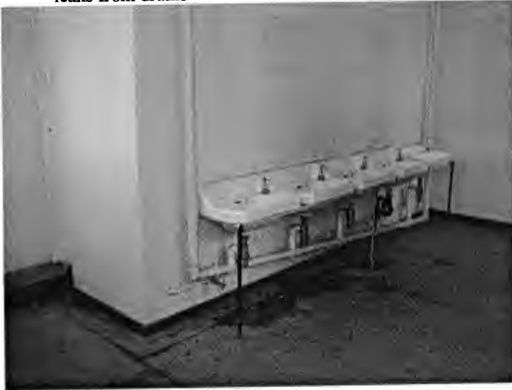
Image 45: 04K03b: Highway Secondary: Girls' cloakroom with wall marks where mirrors once were, and leaks from drains
