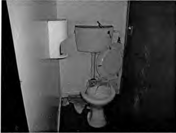
Image 144: 06K03f: Simunye Secondary: Vandalised toilet
