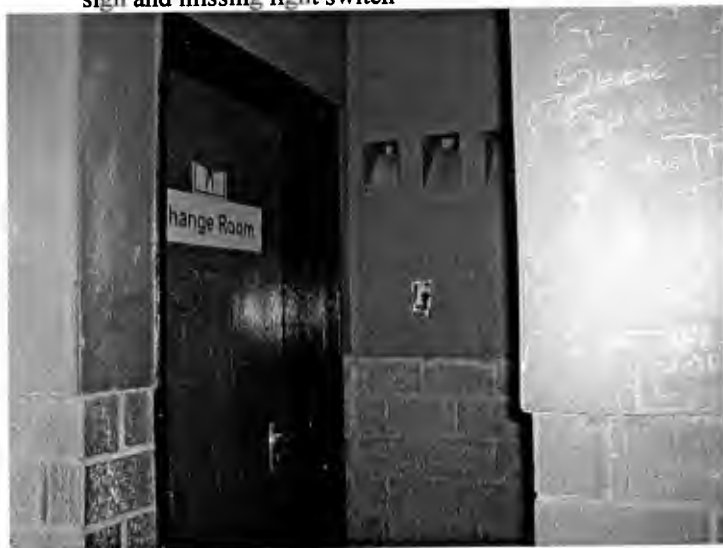
Image 142: 06Kgraffiti02 : Simunye Secondary: Boys' change room entrance showing graffiti, broken sign and missing light switch
