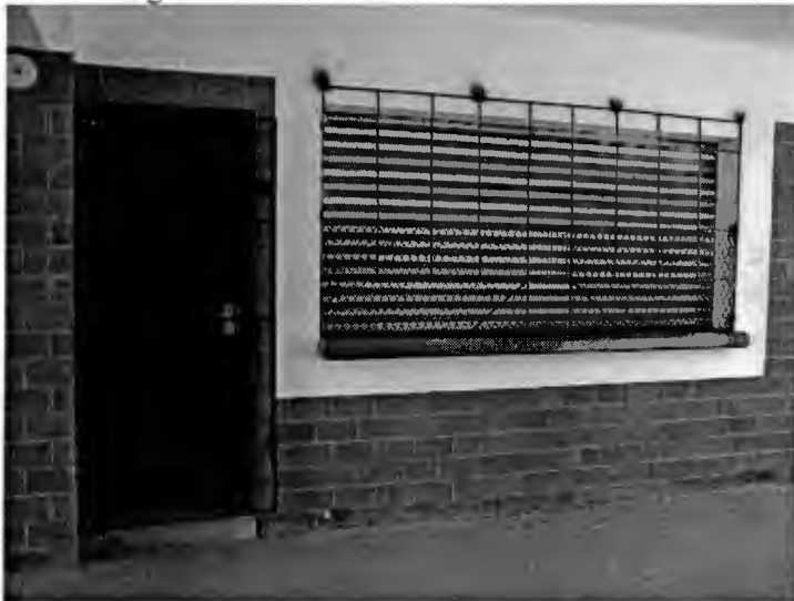
Image 145: 06K23b: Simunye Secondary: Tuckshop showing roll-down shutter and new security bars with welding burn marks
