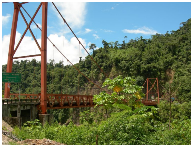
Figure 1. The Inambari Bridge, where the Interoceanic Highway crosses the River Inambari. Source: authors.
