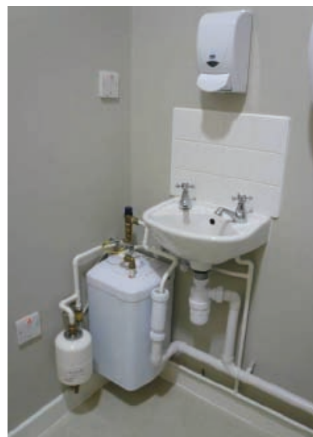
Complicated services which are badly integrated do not contribute well to environmental sustainability
