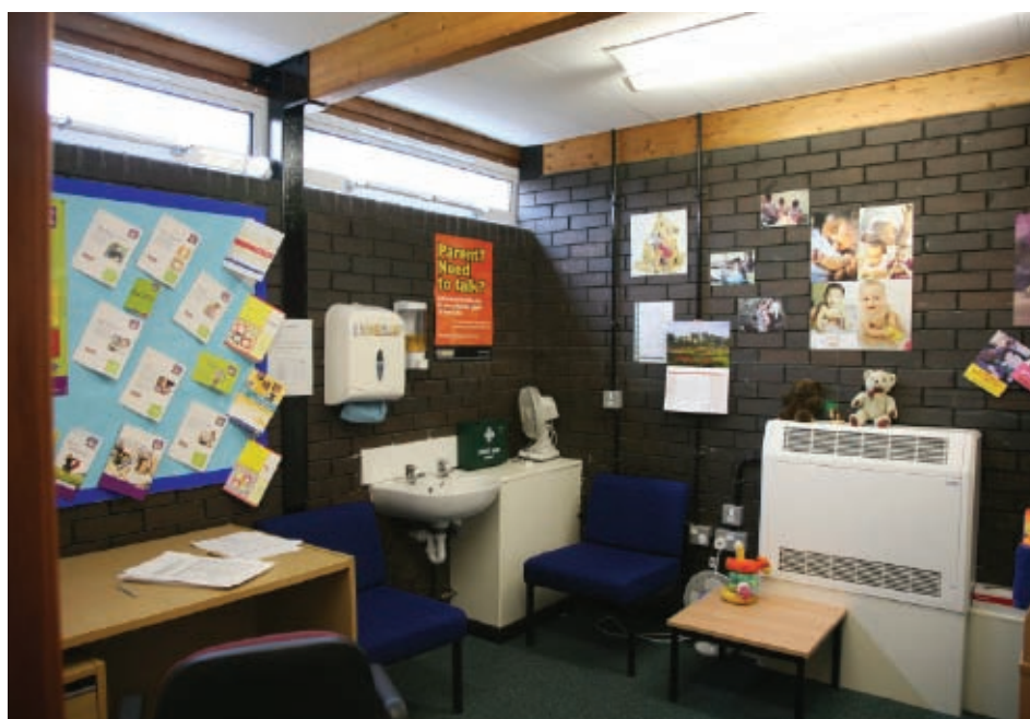
High windows offering less light and no views mean that artificial lights are kept on all day and spaces seem smaller, darker and unanimated
