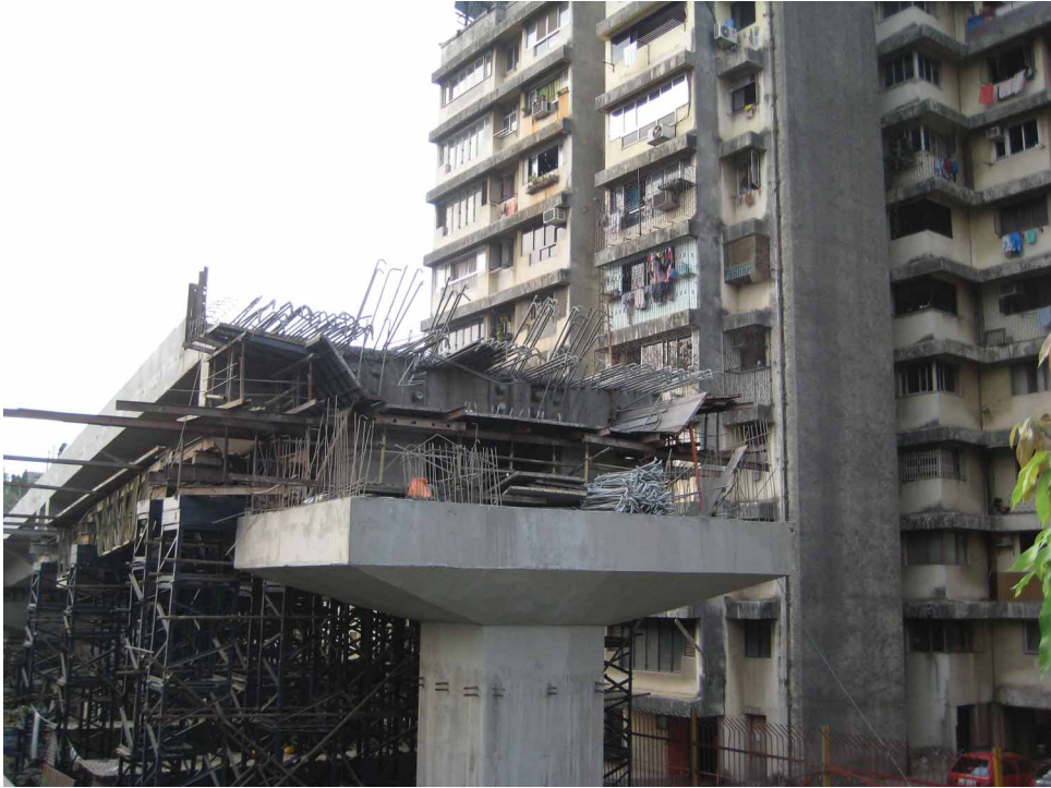
Figure 10 Unfinished flyover at Barfiwala Lane, Andheri West, April 2009. Photograph by the author.
