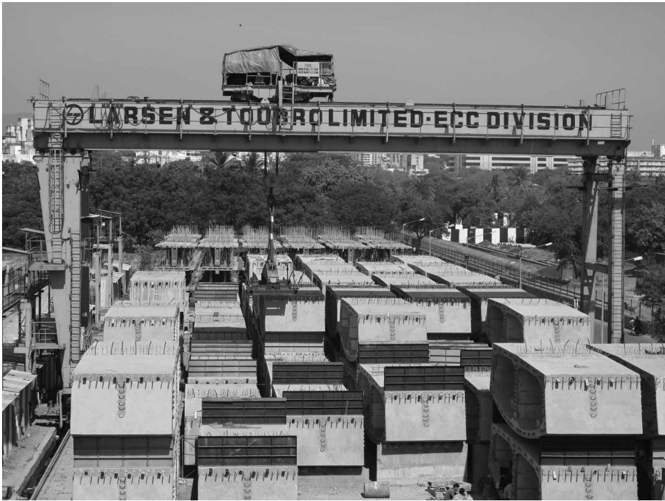
Figure 1 Concrete casting yard for the Sahar Elevated Road, in the vicinity of Chhatrapati Shivaji International airport, December 2009. Photograph by the author. Please visit www.verticalurbanism.com for further visual material
