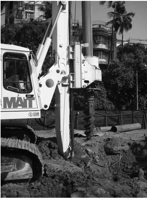
Figure 4 Mait piling equipment from the USA used in the construction of the flyover along Dr Babasaheb Ambedkar Road between Sion and Byculla, April 2009. Photograph by the author.
