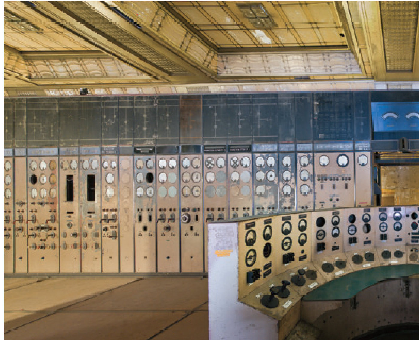
429. Battersea Power Station, Station 'A' Control Room in 2011
