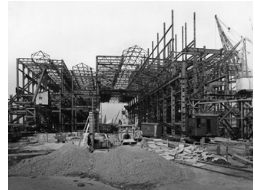
424. Battersea Power Station, steel frame of Station 'A' under construction by Sir William Arrol & Co. Ltd, c.1931
