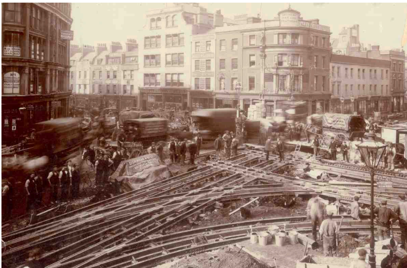
575. Tramlines being laid at junction of Goswell Road and Old Street, 1906. The tall building left of the Hat and Feathers is Stockall & Sons' clock and watch factory at Nos 6–10 Clerkenwell Road
