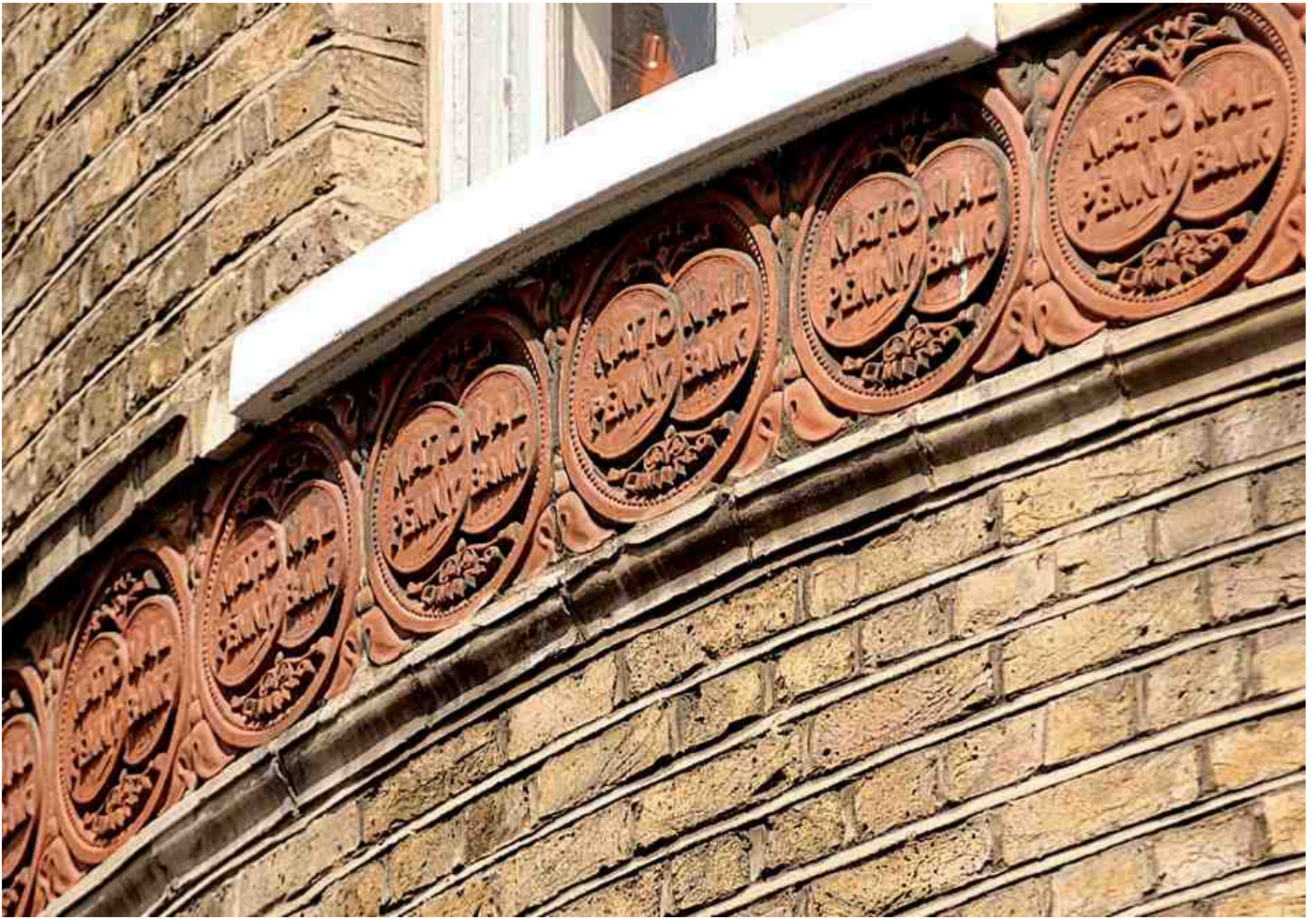
559, 560. Pennybank Chambers, Nos 31–33 Clerkenwell Road and 33–35 St John's Square, in 2006. Charles Henman and William Harrison, architects, 1879–80
