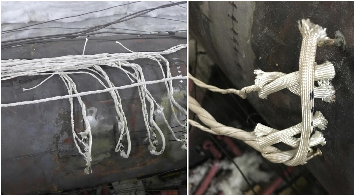
Figure 4. Left – Stud connections after installation on horizontal vessel, Right – close up of a set of 6 studs, the outer two for the excitation current and two inner pairs for the signal from each HAZ
