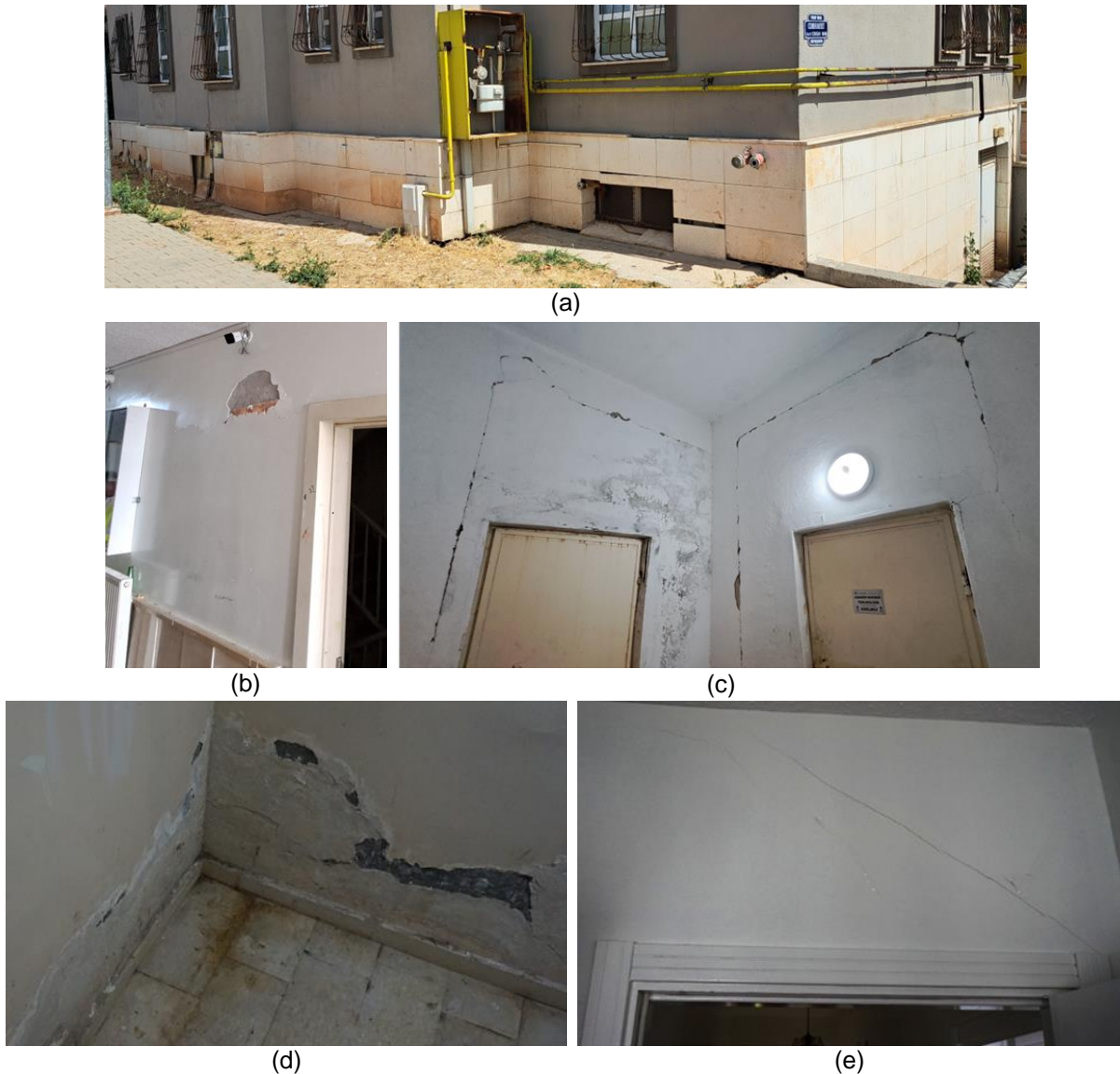
Figure 4. Damage patterns of high-rise tunnel-form building in Nizip. a) Damage to the façade elements; b) Spalling of plaster; c) Separations between the infill walls and structural elements; d) Damp in the basement floors; e) Onset of diagonal cracks in a coupling beam.
