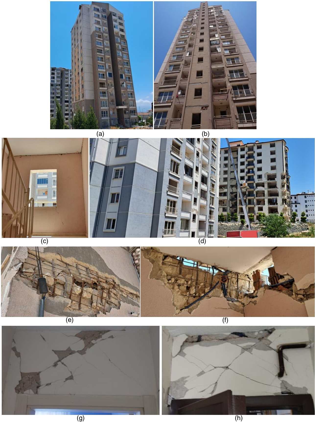
Figure 6. Damage patterns of high-rise tunnel-form building in Antakya. a) Front of the building; b)Rear of the building; c) Separation of the infill walls from the structural system; d) Damage to infill walls in a nearby tunnel-form building and an RC frame; e) Damage to shear wall, exterior view; f) Damage to shear wall, interior view; g) Diagonal cracks in a coupling beam; h) A commonly observed construction flaw.
