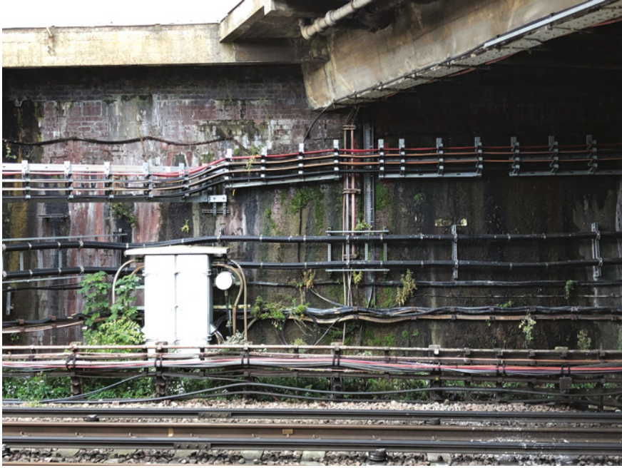
FIGURE 11.10 Synthetic biotope – leaking wall with biofouling at Preston Road Station, London, 2021
