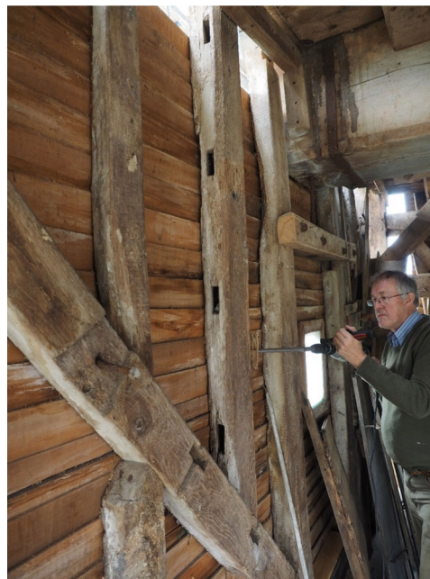
Figure 17. Two pre-used old timbers that were upcycled during a past rebuild into wall studs in the buck wall at Great Chishill Windmill. Martin Bridge is drilling a dendro sample from one of them, which when analysed showed it was from a tree felled in the period 1693–1726 (photo: Martin Davies)
