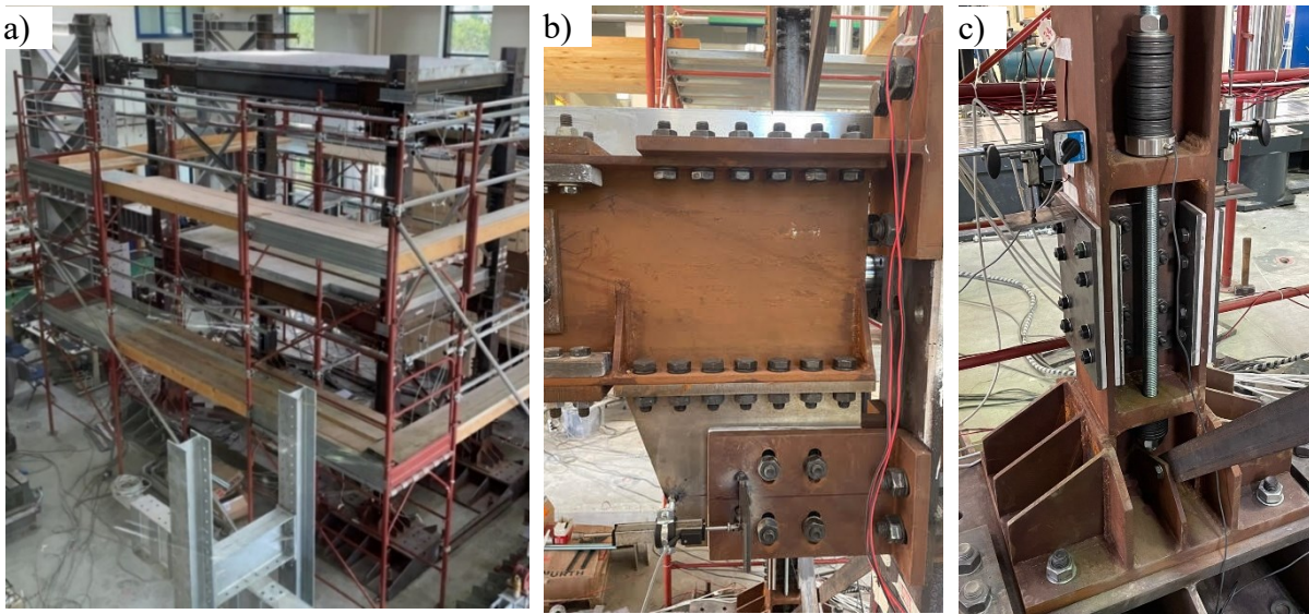
Figure 1: Large-Scale steel tested structure: a) Tested structure; b) FREEDAM beam-to-column connection; (b) SC-CB connection.
