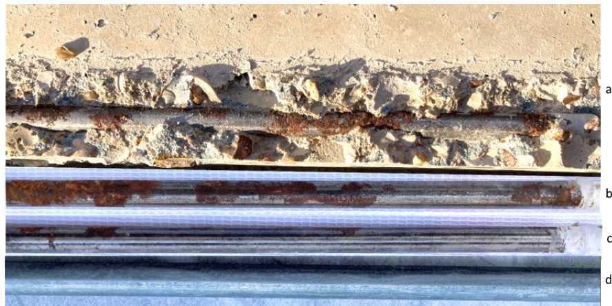
Fig. 6.17 The amount of rust formed on the surface of the rebar in specimen type B made of FA: (a) the visual appearance of the specimens after the splitting into halves; (b) the surface of the rebar facing the crack, (c) the side away from the crack (d) the surface of the reinforcement facing the crack after the picking
