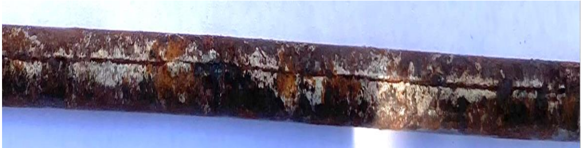
Fig. 6.22. The appearance of V-shaped pitting corrosion formed along the crack in Specimen design C.
