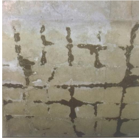
Fig. 3.2 Plastic shrinkage cracks follow the pattern of the reinforcement (Concrete Society, 2010).
