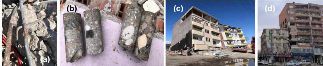
Figure 4. Damage representations from the earthquake-affected cities (a) Plain round rebars and 90° hooks at the end of stirrups, (b) Abnormal granulometry, (c) Soft/weak story, and (d) Pounding effects
