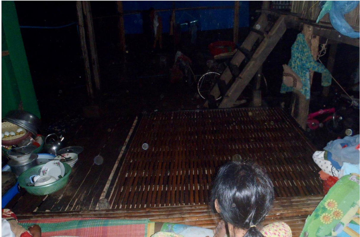
8. Photograph showing Saatchi's mother looking at leaks in their house. © Waan, Village B.
