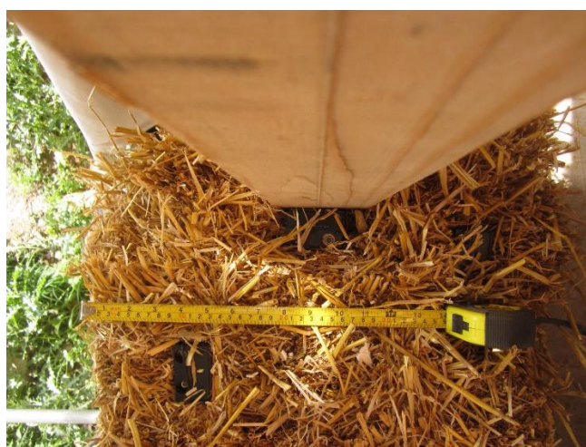
Fig. 2. Outer sensor (left) and central sensor (centre) installed in the strawbale wall.
