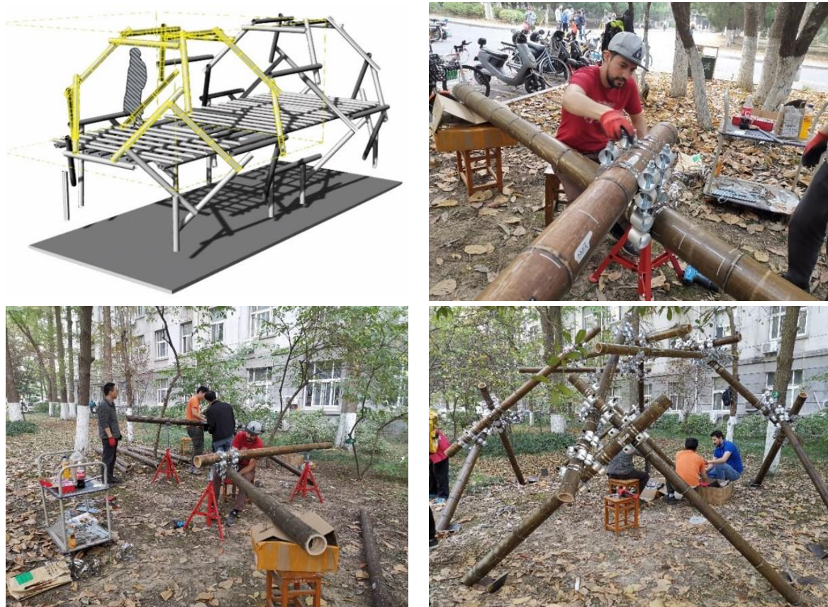
Fig. 1. Future bamboo housing – case study of 2019 China-UK international collaboration in bamboo structure practice (credit: Haitao Li, Rodolfo Lorenzo).
