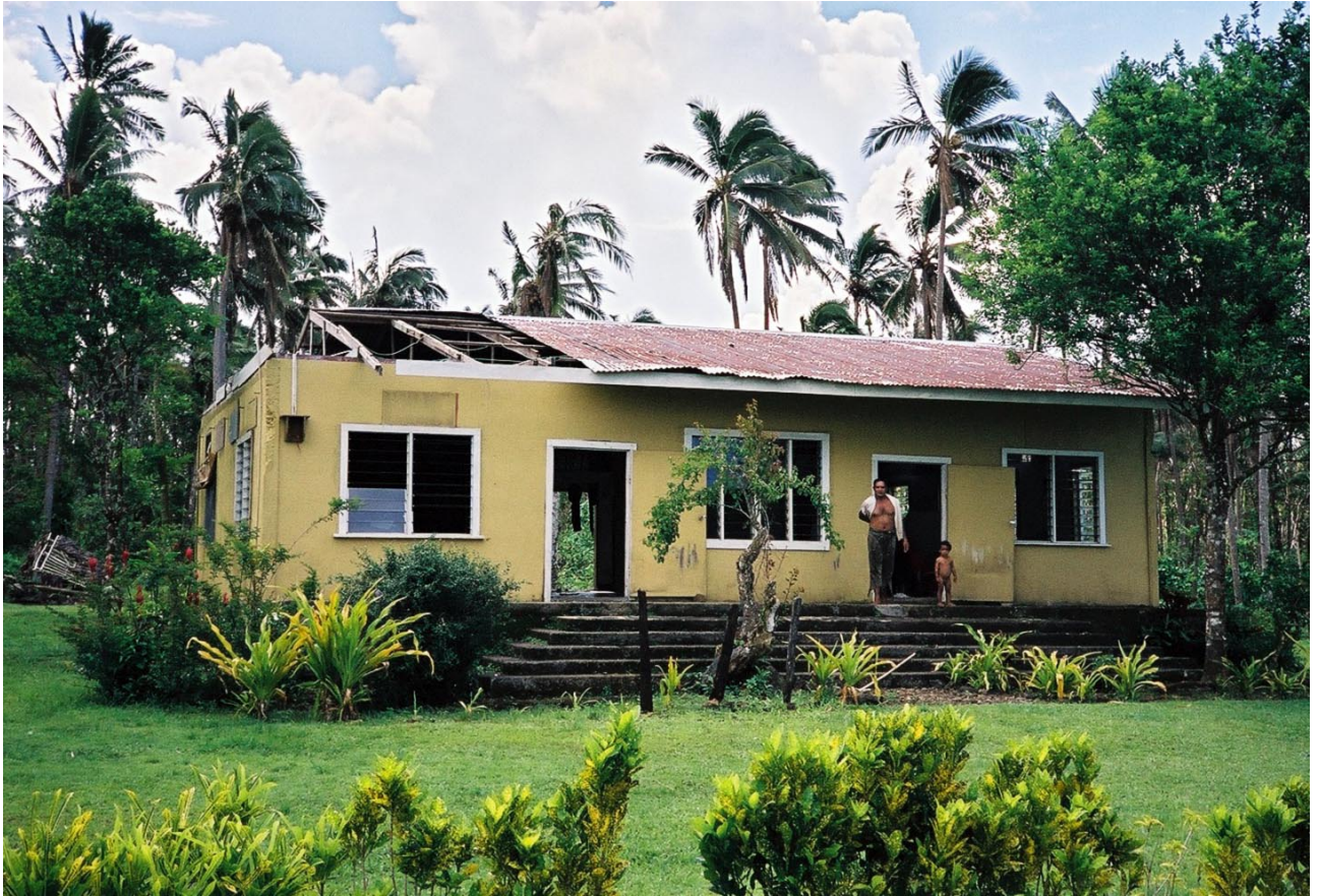
FIGURE 11. A Samoan family's damaged roof
