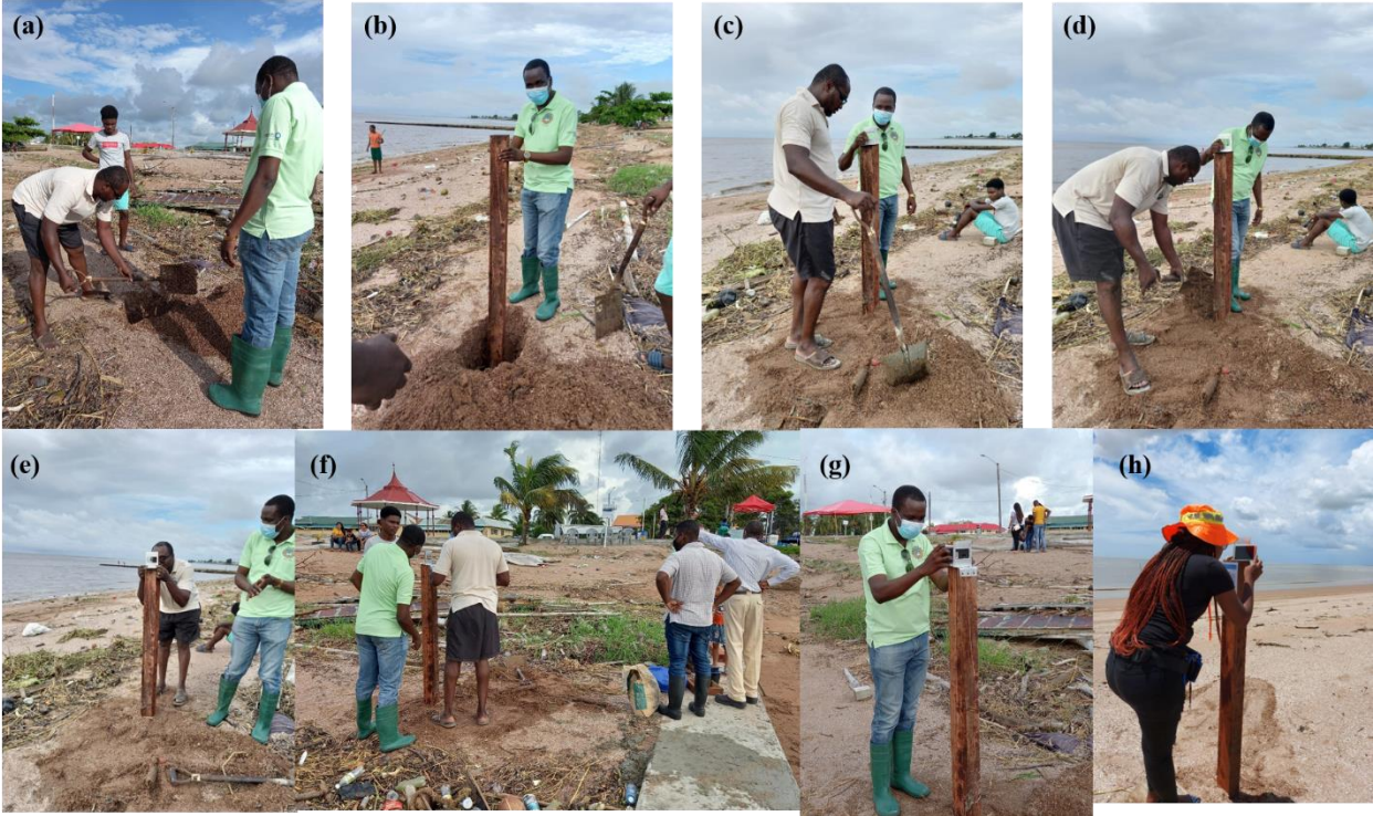
Figure 4 The processes of erection of the photoposts at one of the sites (a – e), staff from the Ministry of Public Infrastructure were on the ground to observe the erection and to ensure that where the permission was given is where the posts are erected (f), erected posts at bandstand side (g) and another post at behind Marriot (h) with Joy taking the first set of pictures from the location
