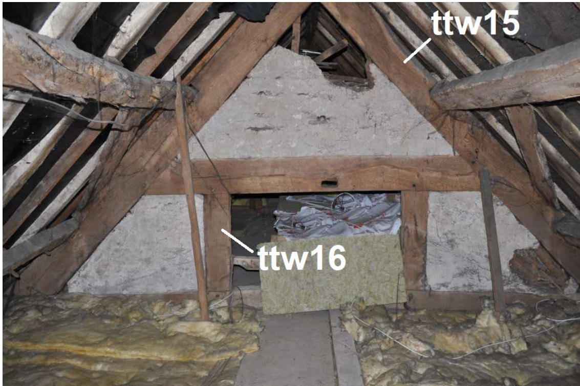
Figure 7: View of truss 10 looking south, showing timbers sampled for dendrochronology (photograph Duncan James)
