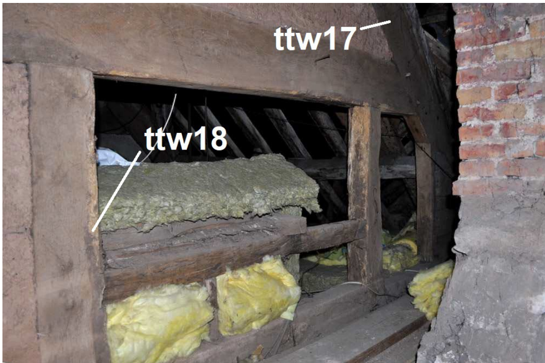
Figure 8: View of truss 11, looking north, showing timbers sampled for dendrochronology (photograph Duncan James)
