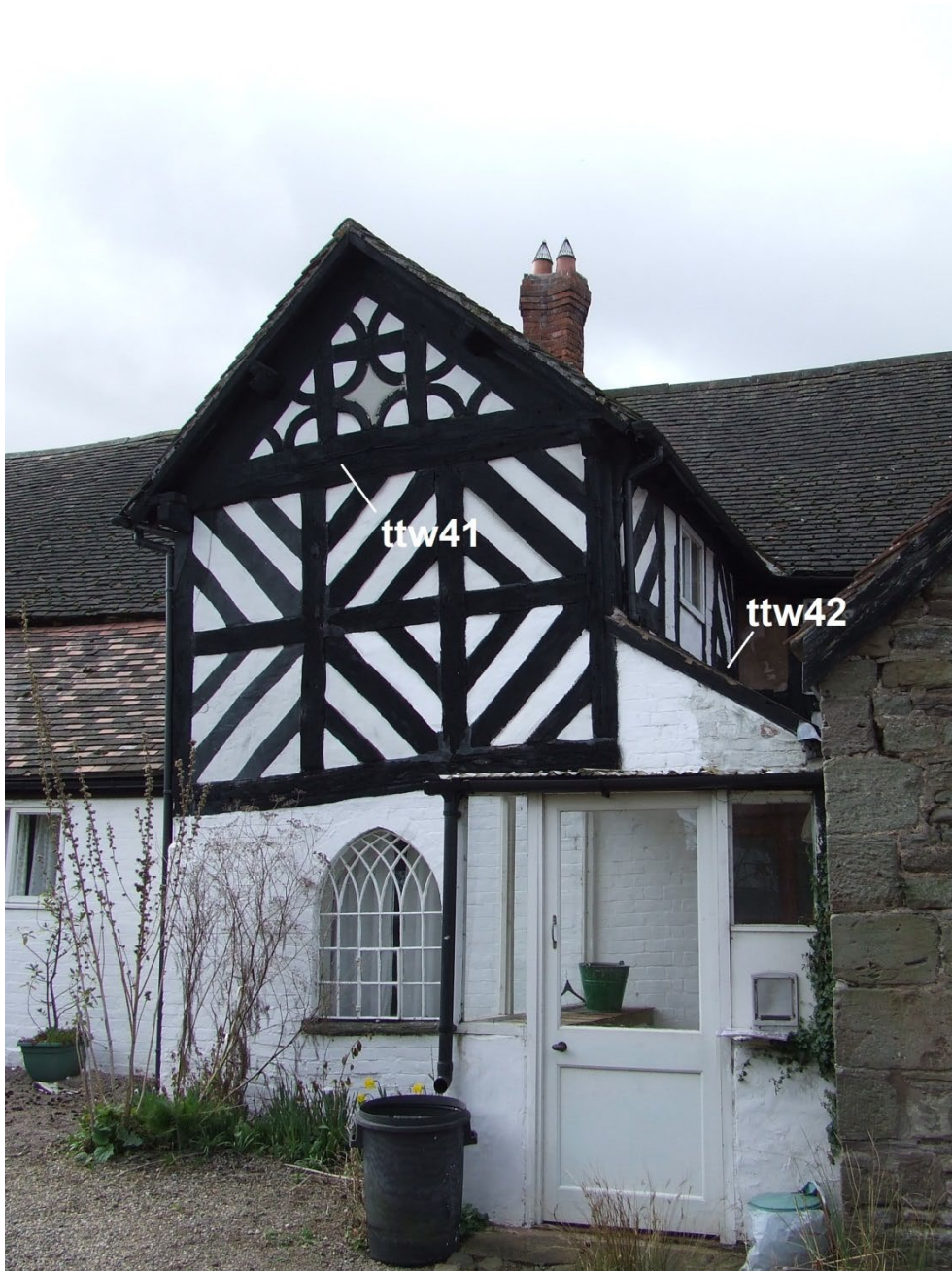
Figure 4: View of the porch, looking south-west, showing the tiebeam and mid-rail sampled for dendrochronology (photograph Martin Bridge)
