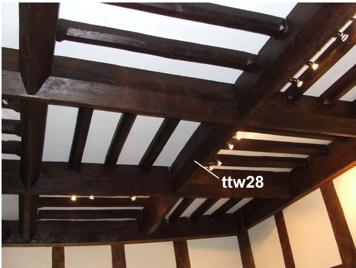
Figure 12: Ceiling of the ground-floor room in bay 7, looking east, showing the beam sampled for dendrochronology (photograph Martin Bridge)
