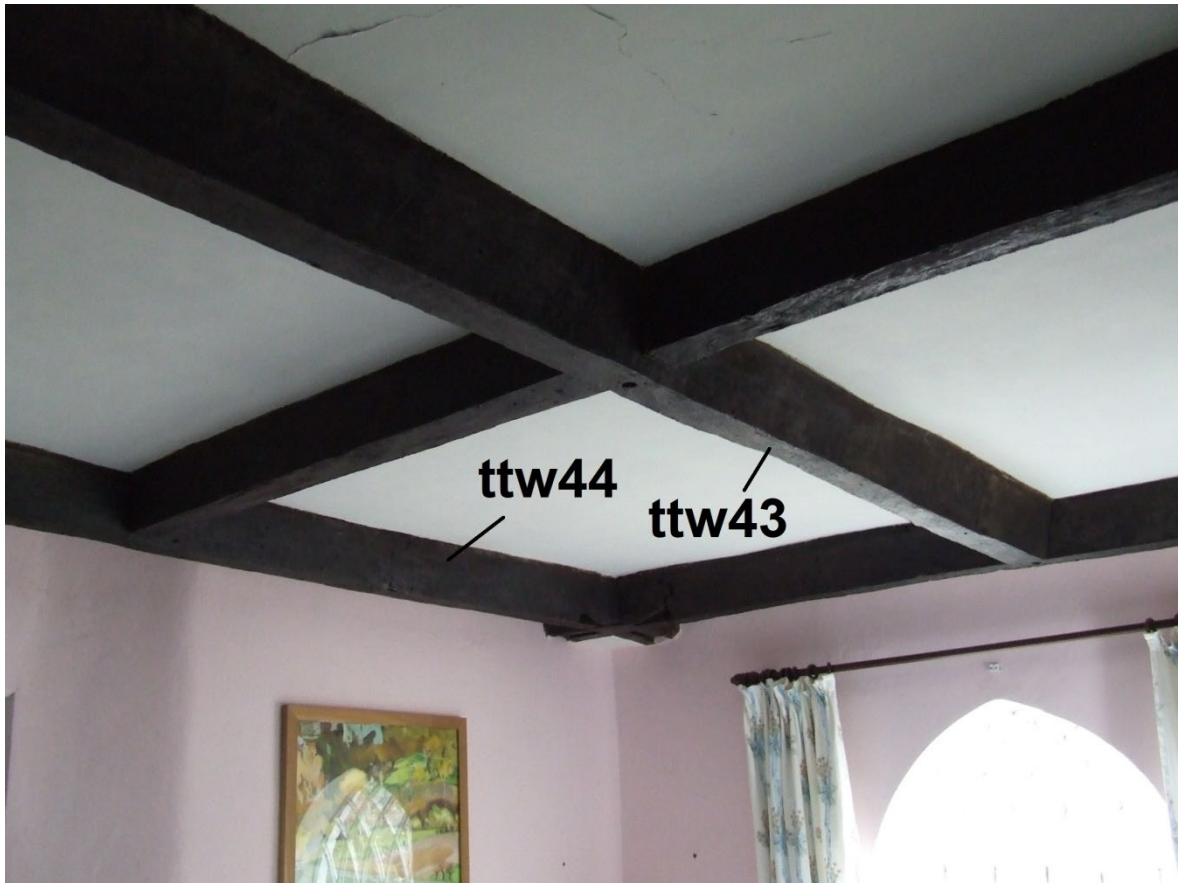
Figure 13: View of the porch ground-floor ceiling, looking north-east, showing the beams sampled for dendrochronology (photograph Martin Bridge)
