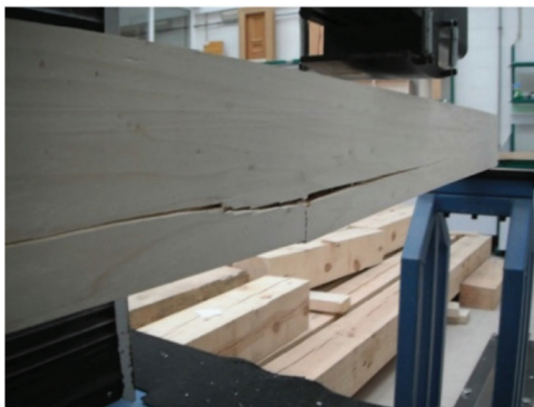
Figure 11: Failure mode of 1200 g/mm 2 GFRP reinforced beams [64]
