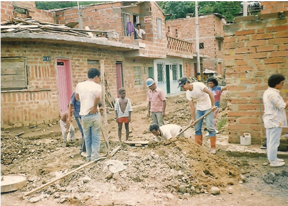
FIGURE 3 Building a road through a convite in Moravia (source: Community Archive, Moravia Cultural Center, reproduced by permission of Centro de Desarrollo Cultural Moravia)
