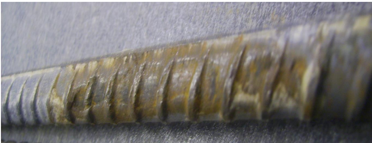
(b) PC - corrosion spread over a larger region
