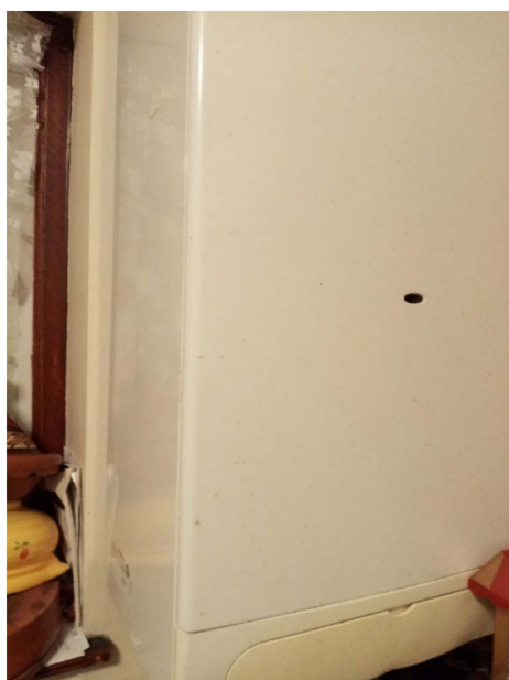
Figure 19. "Broken boiler. The boiler is not working". Participant.Survey10.
