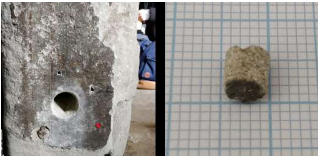
Figure 1. Two examples of coring for \mu CT analysis. Left: example of in situ sampling hole at Hampton Court with a 25.4 mm core sample taken at the centre, surrounded by two 3 mm regular drill holes for drilling resistance measurements. Right: 5 mm diameter core sample taken for \mu CT analysis, showing a black gypsum crust on its surface.
