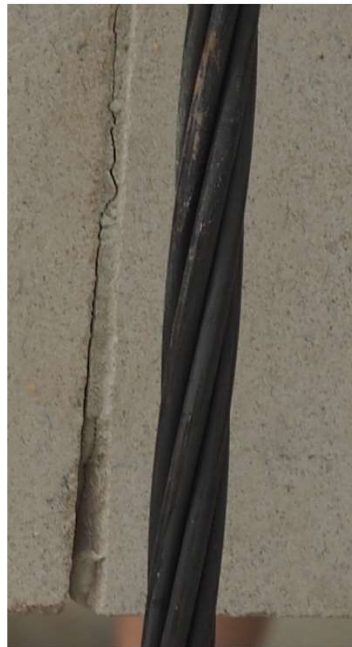
(c) Separation (crack) at mortar-stone interface at midspan
