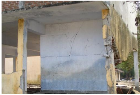
Figure 12. Shear failure observed in a corner column of a typical school building after the 2004 tsunami.
