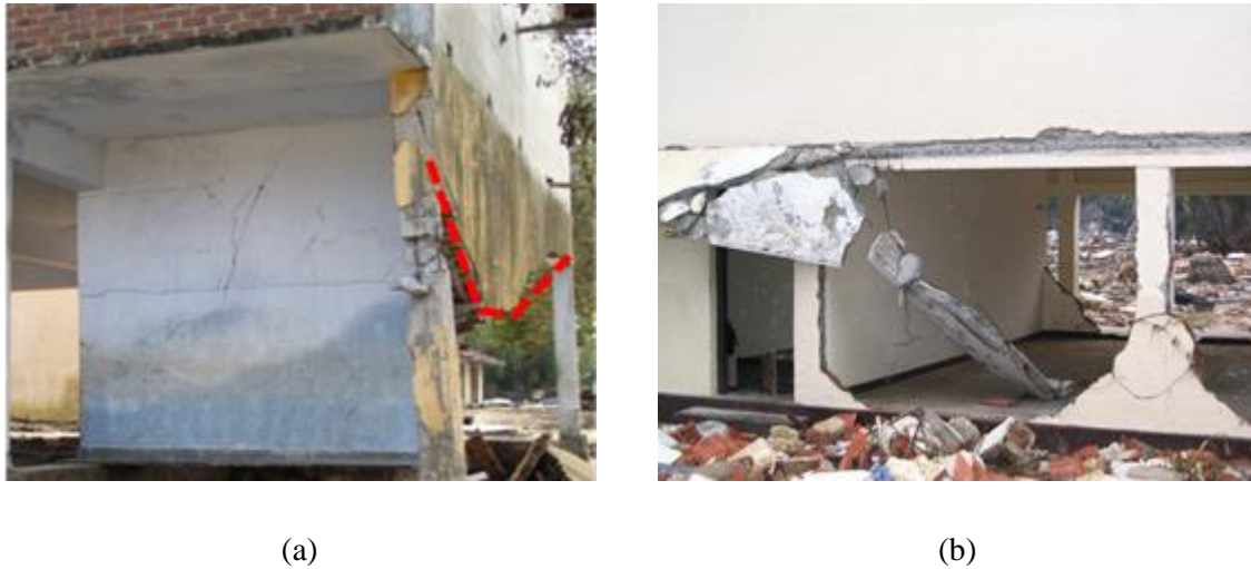
Figure 8. Out of plane failure modes observed in infill walls of school buildings in Sri Lanka under the 2004 Tsunami: (a) tsunami mainly acting along the x direction, and (b) tsunami mainly acting along the y direction.
