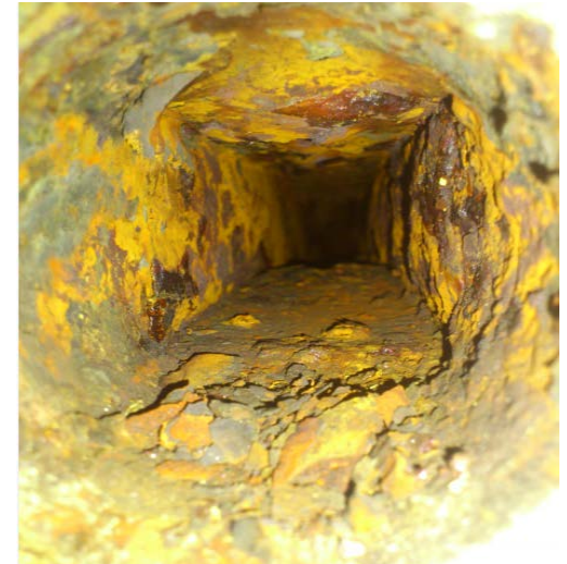
Detail of pipe between ID and RC Fan
