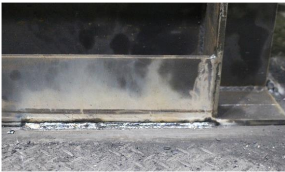
Figure 14. A 300 mm long welding of a supporting jig along part of the furnace boundary.
