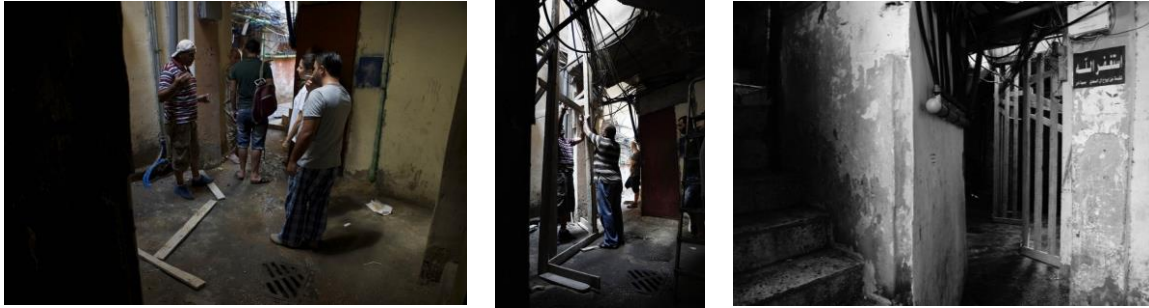
Mode 1: (L) laying out the installation outline whereby extending the existing scale, (C) Constructing the installation, (R) Installation piece acting as another element within the larger camp-apparatus.
