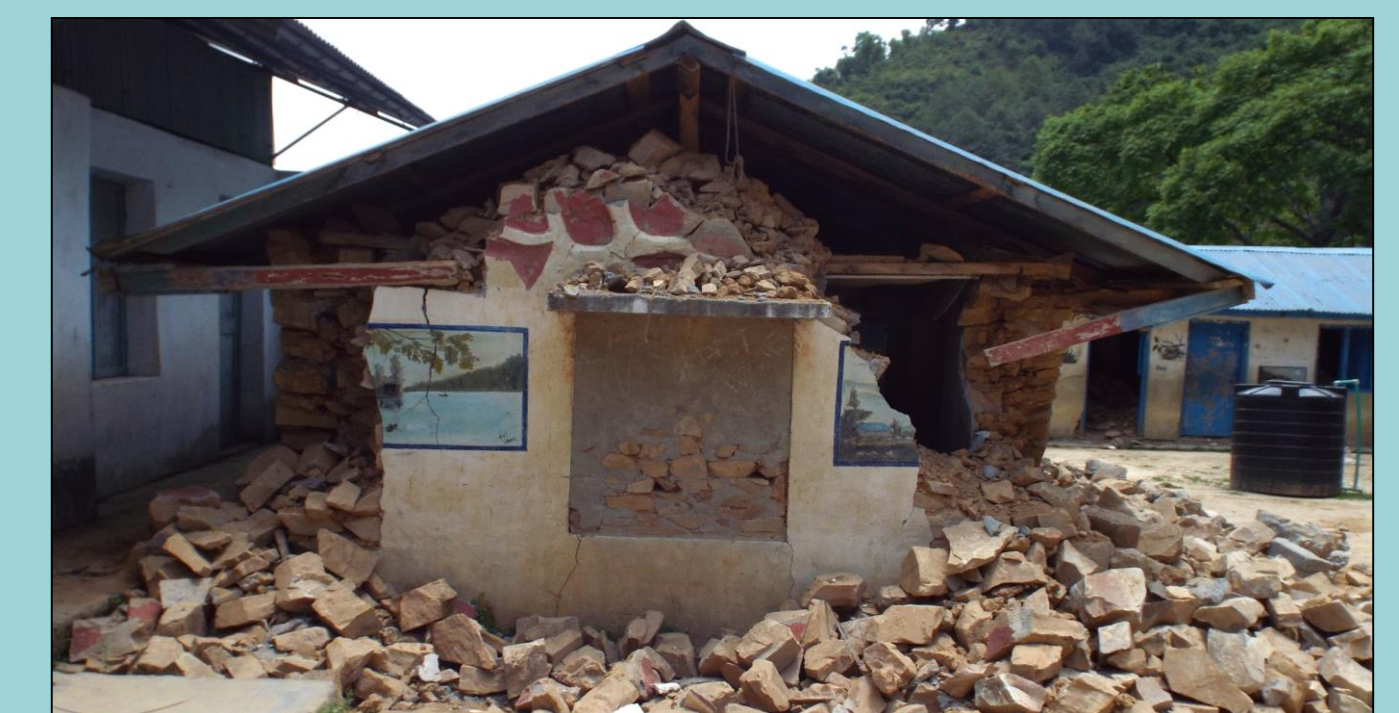
Figure 2: A stone in mud masonry school building damaged due to the 2015 Gorkha earthquake.
