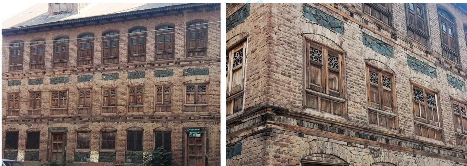
Fig. 3. Referred to as Taqq construction. This system of architecture was prevalent during nineteenth-century consisting of load-bearing masonry piers and infill walls with wood "runners" at each floor level used to tie the walls together with the floors.
