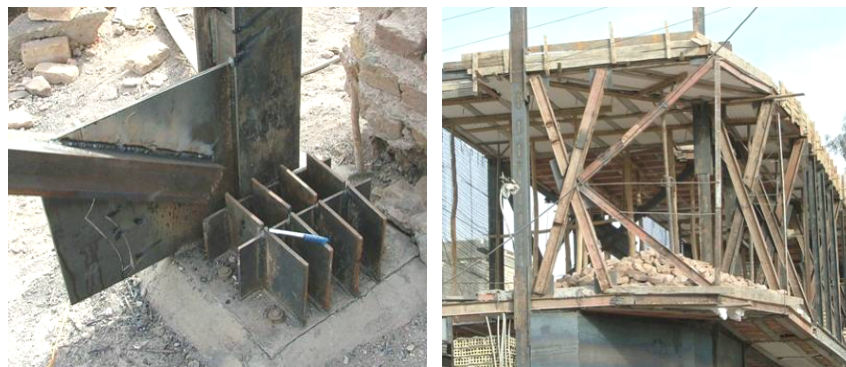
Figure 4: Improper use of reinforcement illustrates the presence of a blind application of safe-construction knowledge (photos by Gharaati)
