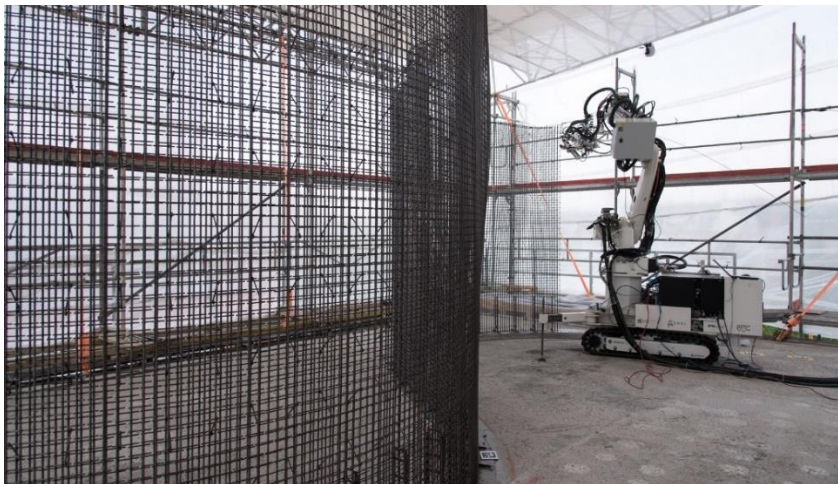
287 288 Figure 6. In situ Fabricator building the Mesh Mould Wall (source: NCCR Digital Fabrication, 2017)
