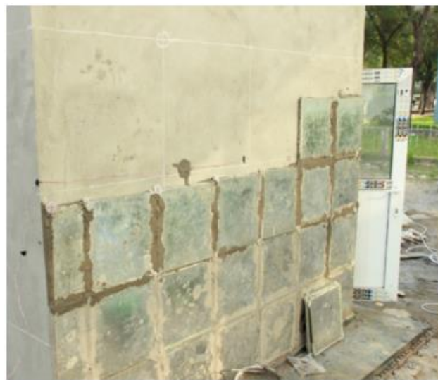
Fig.6 Demonstration of PCM panels installed for the PCMOW [99].
